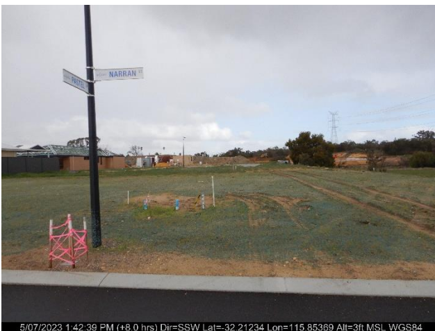
Photo ID: Photo 3 Looking at the cleared lots ready for construction to commence and the road.
