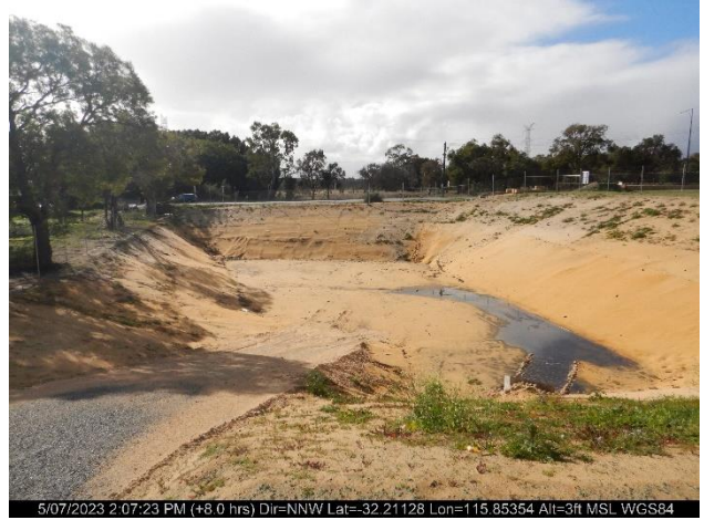
5/07/2023 2:07:23 PM (+8.0 hrs) Dir=NNW Lat=-32.21128 Lon=115.85354 Alt=3ft MSL WGS84 Photo ID: Photo 6 Looking at the drainage sump.
